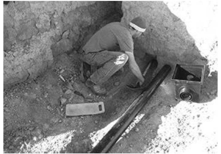
Brian Medchill installing pipe which will lead water away from Mesa Grande wall
