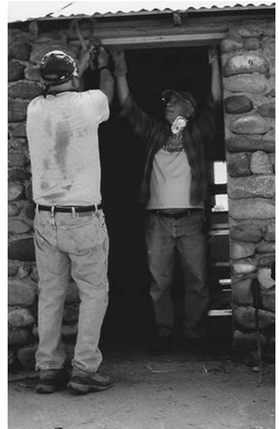
Pat Kelly and Jim Britton installing new door frame at Milk Barn
