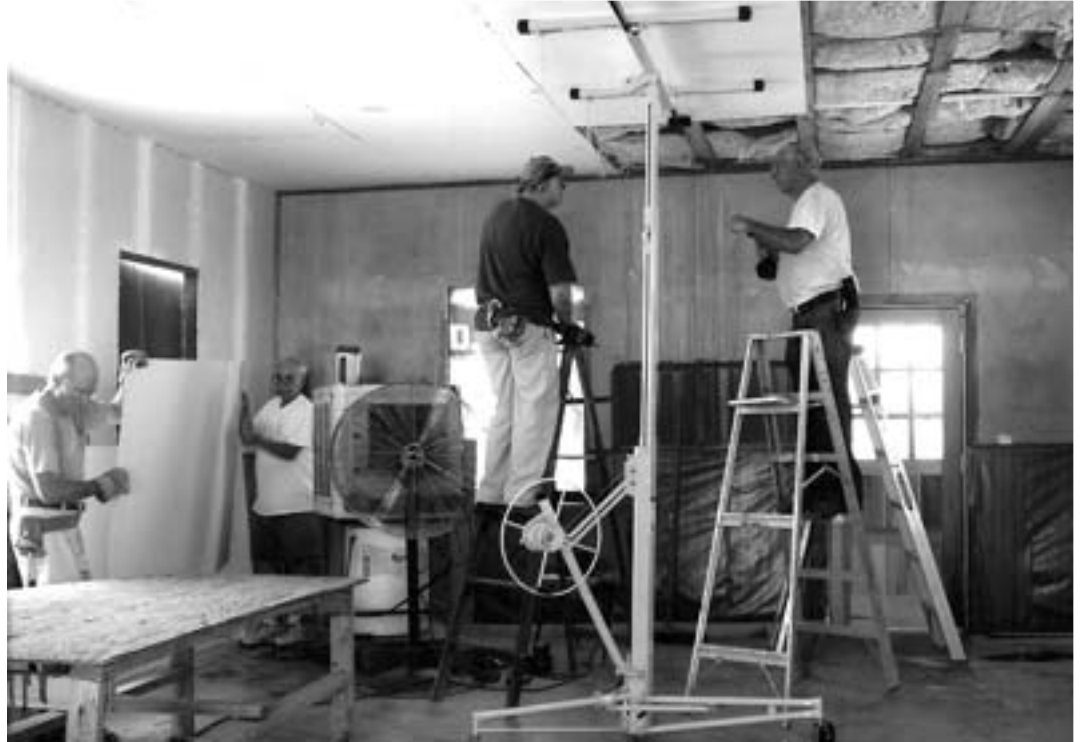
Richard Brown, Jim Britton, KJ Schroeder and Dick Myers use a new mount to hold panel to ceiling. Fans and a swamp cooler helped keep volunteers comfortable.
